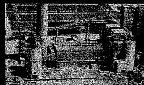
Spray Dry Absorber
