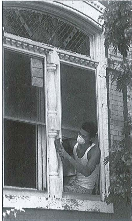
Removing lead-based paint can be difficult and hazardous.
