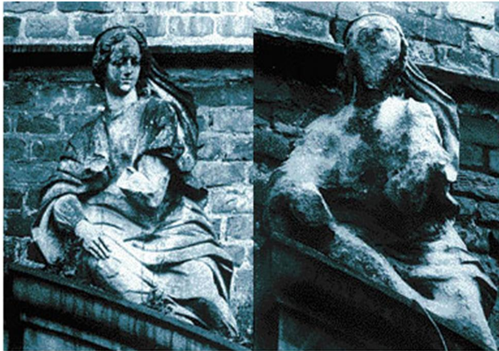
How acid rain affects stonework. The picture on the left was taken in 1908. The picture on the right was taken in 1968
