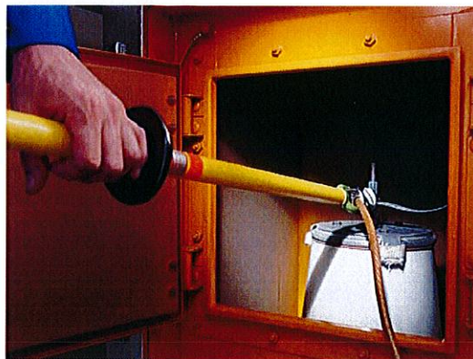
Grounding of insulator
