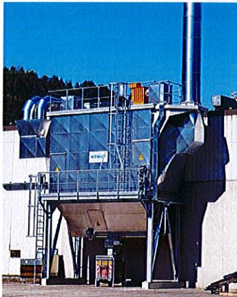
ESP with attached exhaust stack
