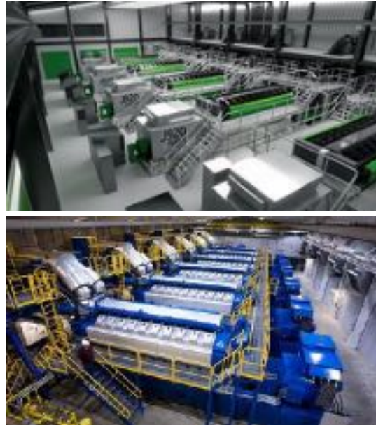
Foto: Fuente Power Engineering International Credit: GE (imagen superior), Wärtsilä (imagen inferior)
