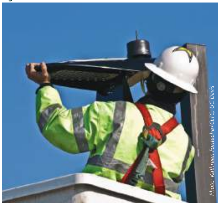
Figure 7. LED luminaire installation at UC Davis
